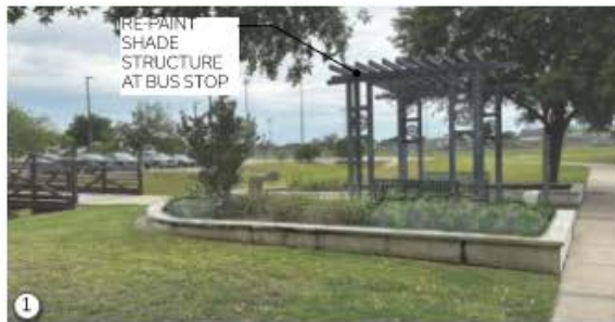
1 RE-PAIN SHADE STRUCTURE AT BUS STOP REMOVE ALL PLANT MATERIAL WITHIN 2FT FROM THE EDGE OF THE PLANTER. WATERPROOF (LIQUID APPLICATION) BELOW COPING ALL THE WAY TO THE FOOTING OF PLANTER. SEAL AND RE-PLANT PLANTERS.
