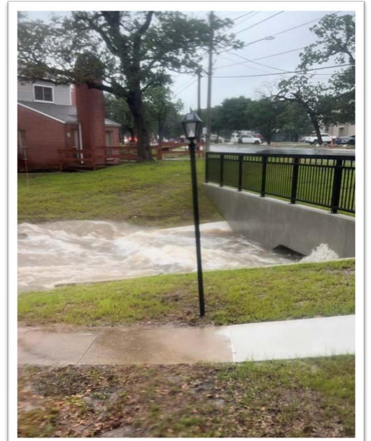
Culverts in action on May 16th
