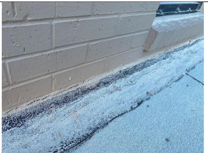
Inadequate roof termination at north elevation low roof (north wing rise-wall)
