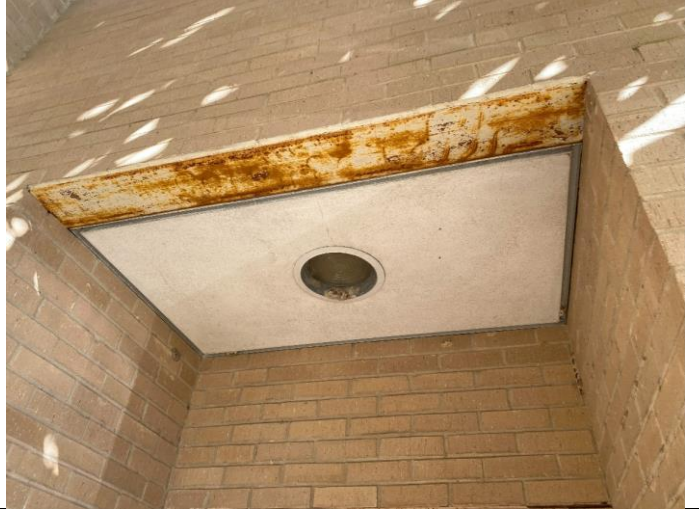
Corroded shelf angle
