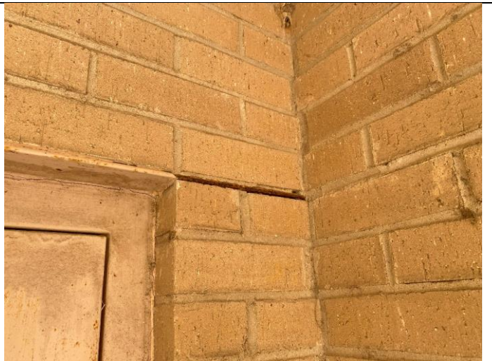
Corroded shelf angle at south elevation (west facing) exit door
