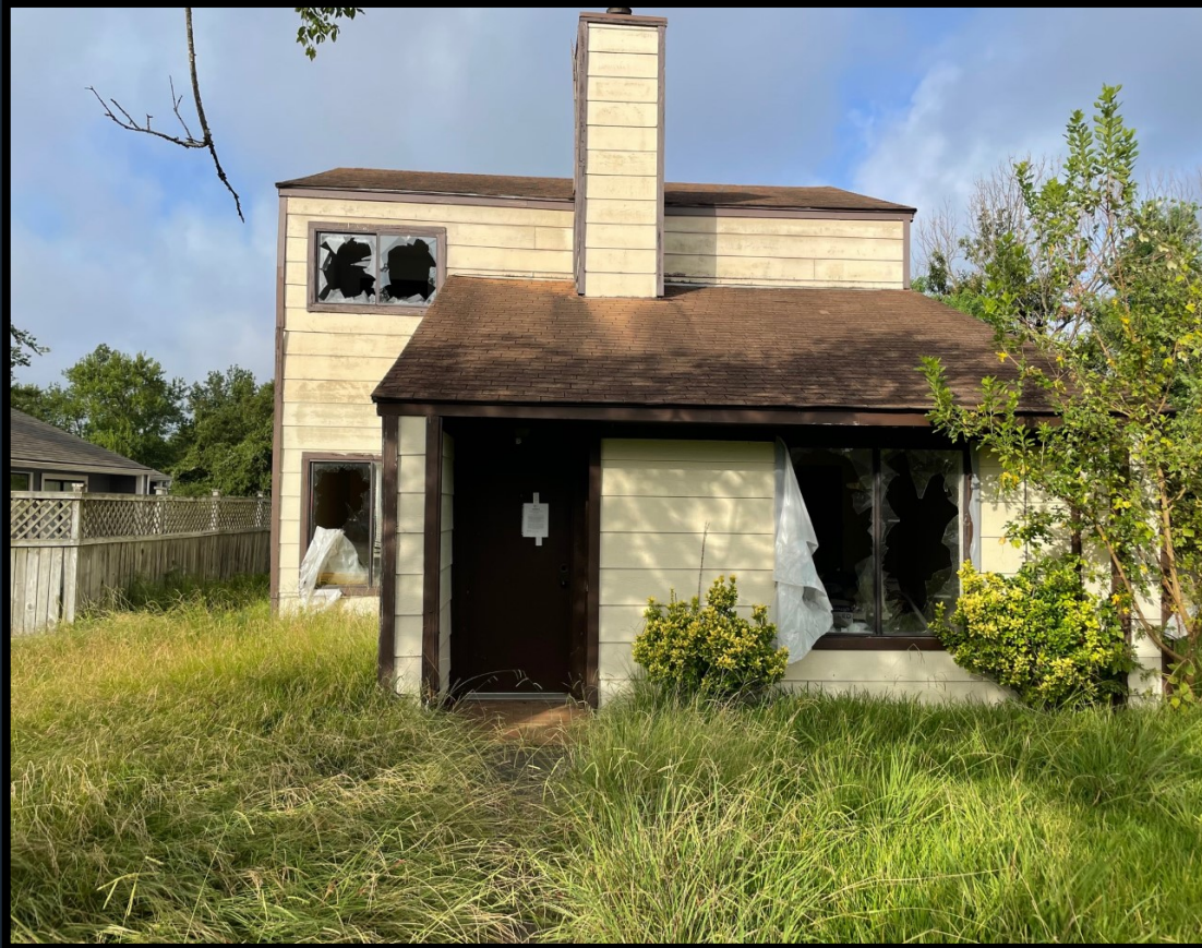
Weeds and Grass/ Unsecured Structure
