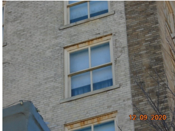
North facing windows still need repairs completed. Rusted lintels, masonry repairs needed, etc.
