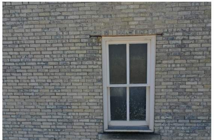
Notes: Rust, no access, interior not observable.
