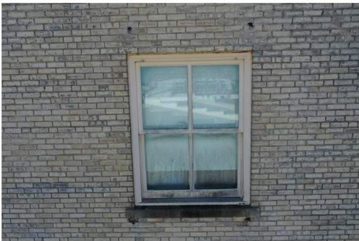
Notes: Rust, brick cracking.
