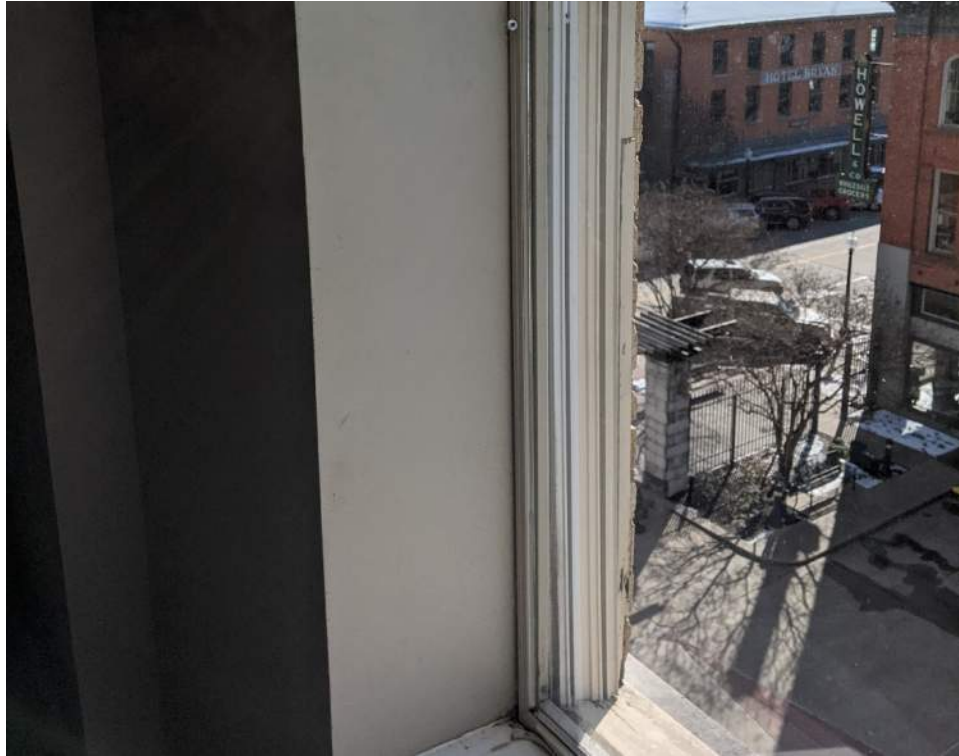
Figure 3 – Example of Inadequate Screw Count
