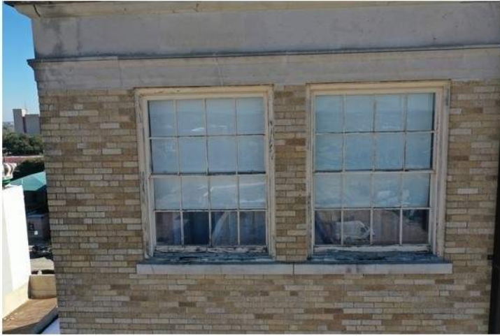
Notes: Wood rot, 7A missing interior storm window.
