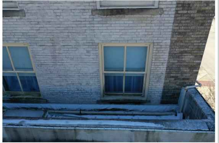
Notes: Storm window, crack in glass.
