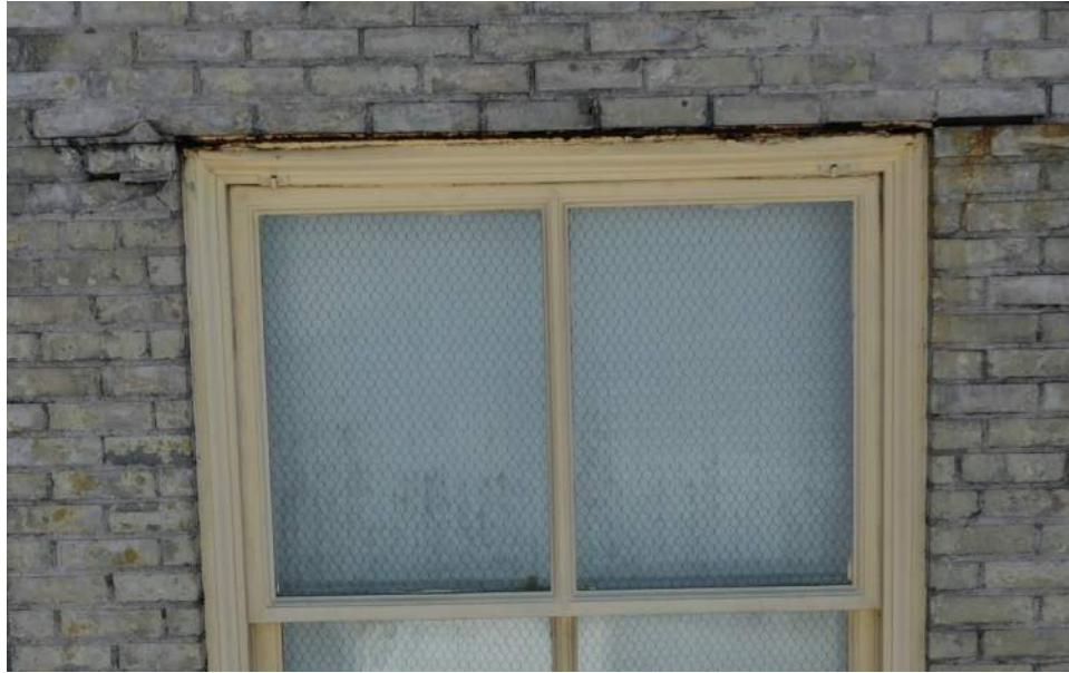
Figure 6 - Example of Minor Cracking Near Lintel, No Signs of Distress Above
