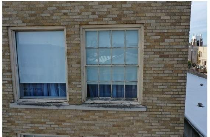
Notes: Wood rot, 4D missing original window sash.
