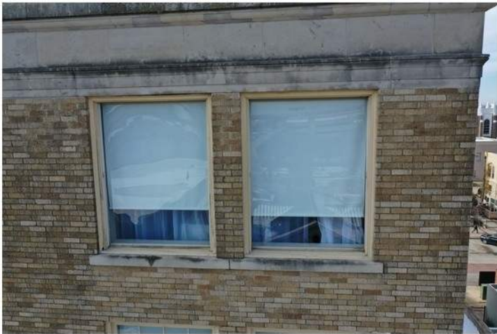
Notes: Wood rot, original window sashes missing.
