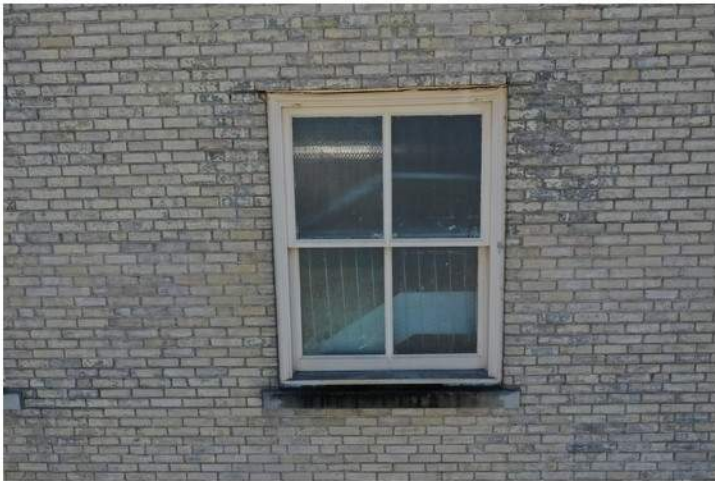
Notes: Rust, brick cracking.
