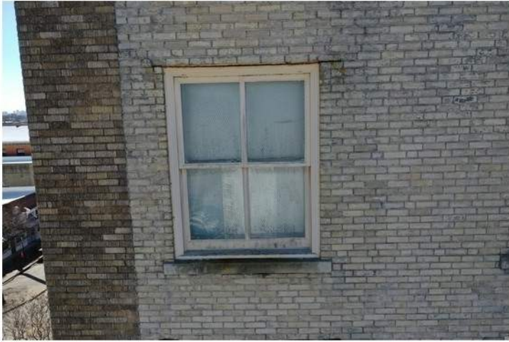
Notes: Rust, brick cracking.
