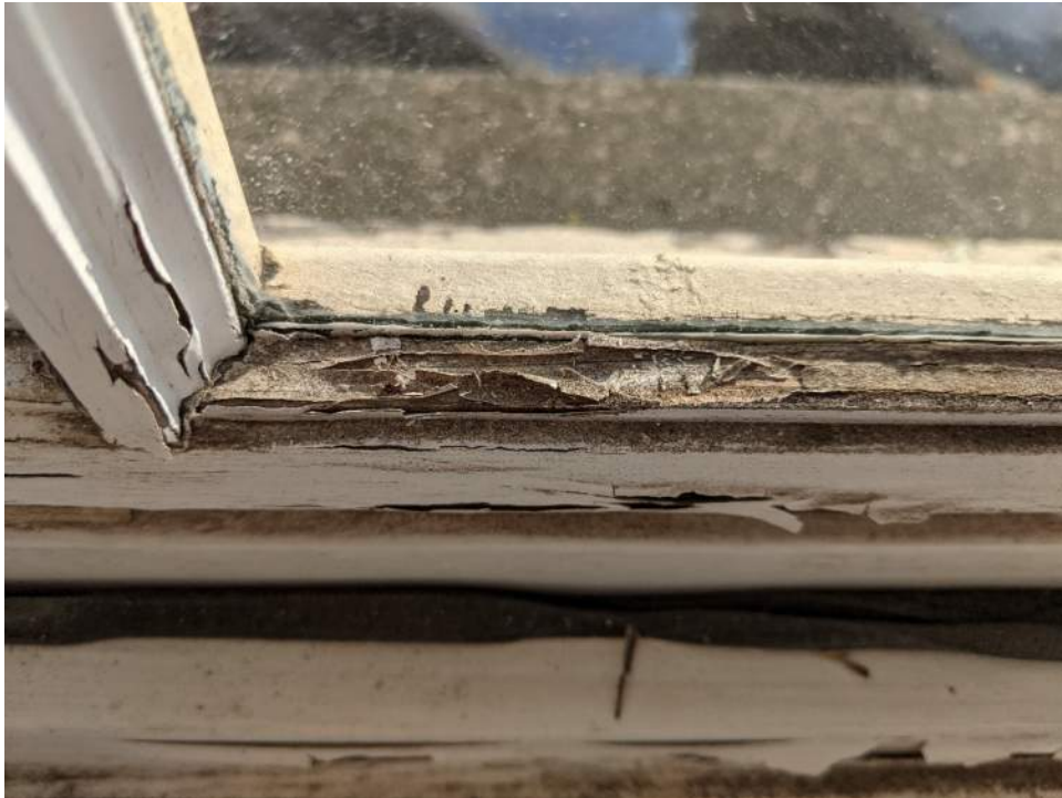
Figure 2 - Wood Rot Penetrating Through Window Sash
