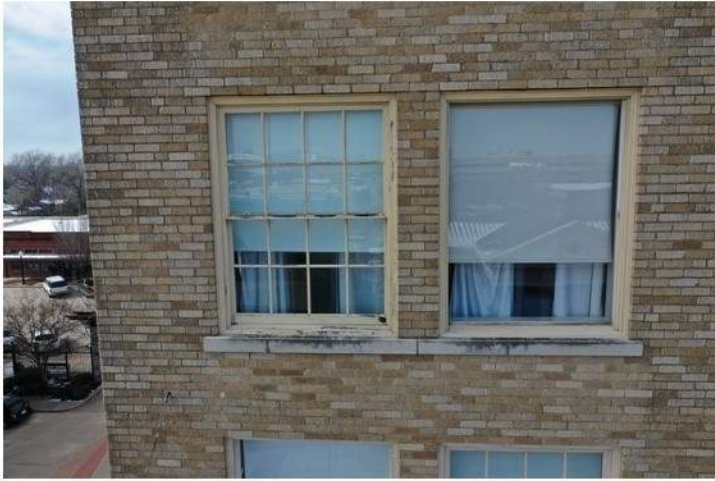
Notes: Wood rot, 5B missing original window sash.
