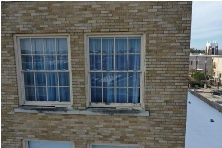
Notes: Wood rot, 5E interior storm window missing.
