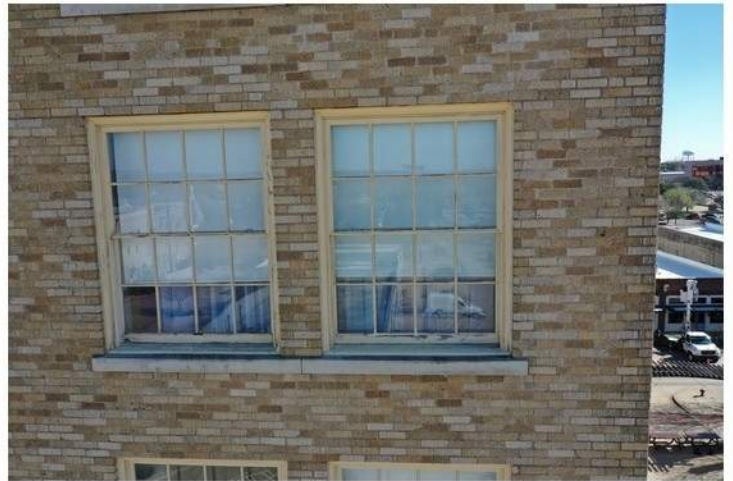
Notes: Wood rot, 6D missing interior storm window.
