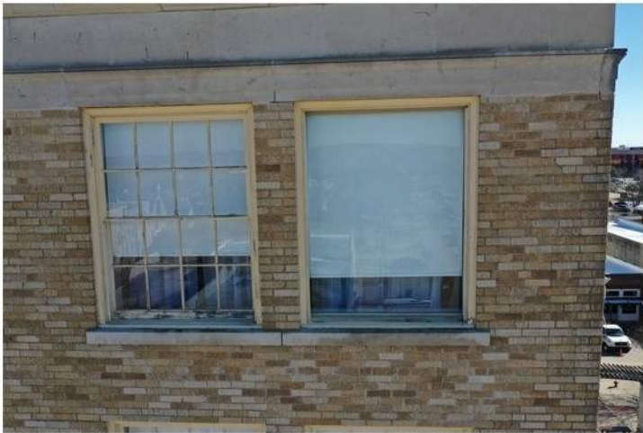
Notes: Wood rot, 7D missing interior storm window, 7E missing original window sash.
