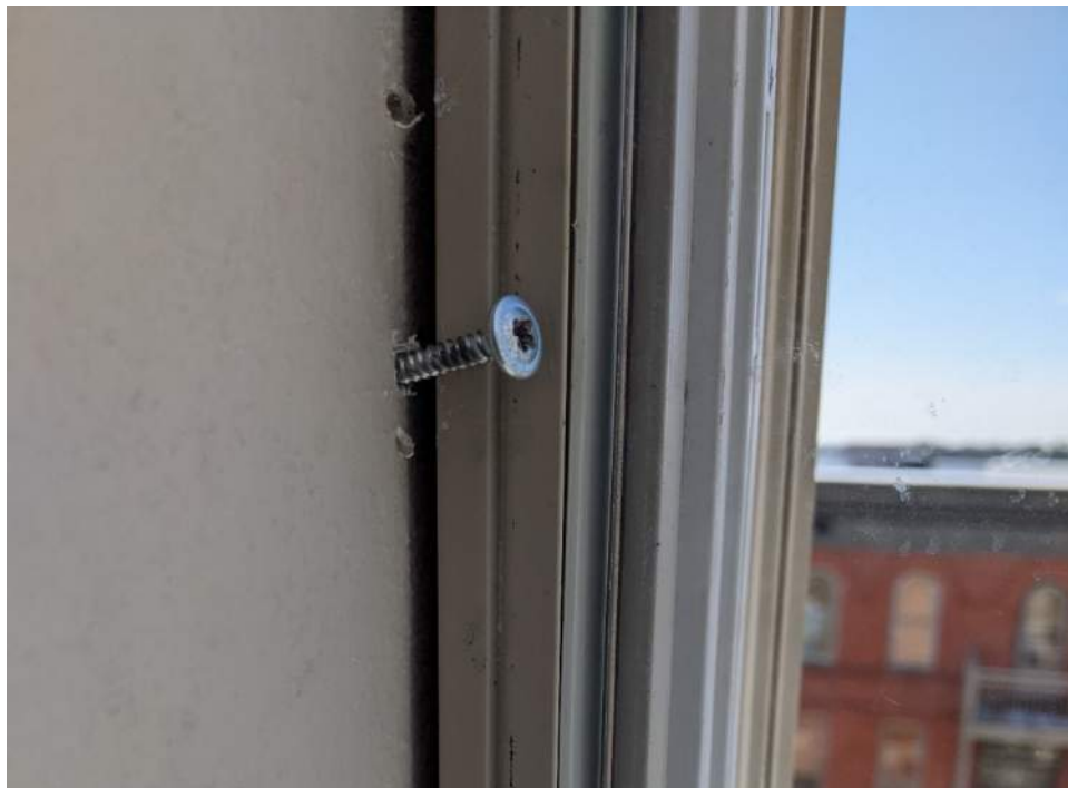
Figure 4 - Example of Screw Missing the Window
