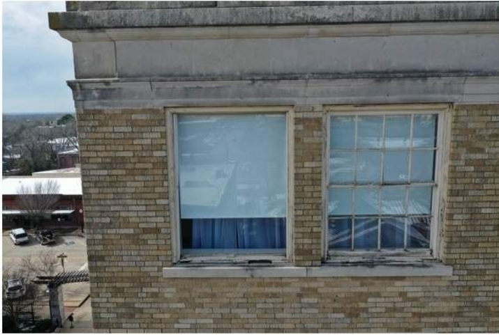
Notes: Wood rot, 7A missing original window sash.
