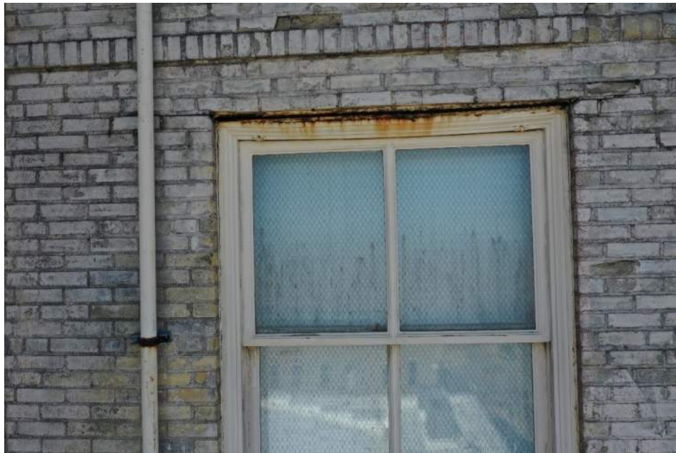
Figure 5 – Example of Rusting at Window Frame
