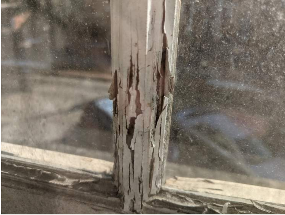
Figure 1 - Wood Rot Penetrating Through Window Sash
