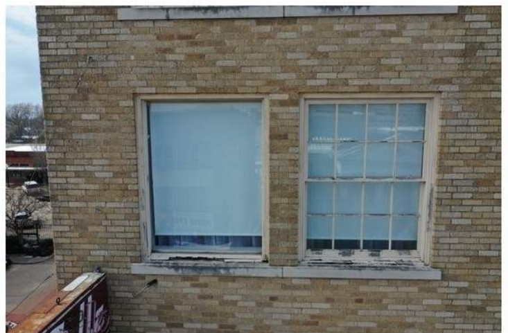
Notes: Wood rot, 4A missing original window sash.
