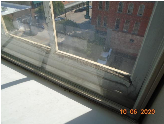
Rot in lower window sash
