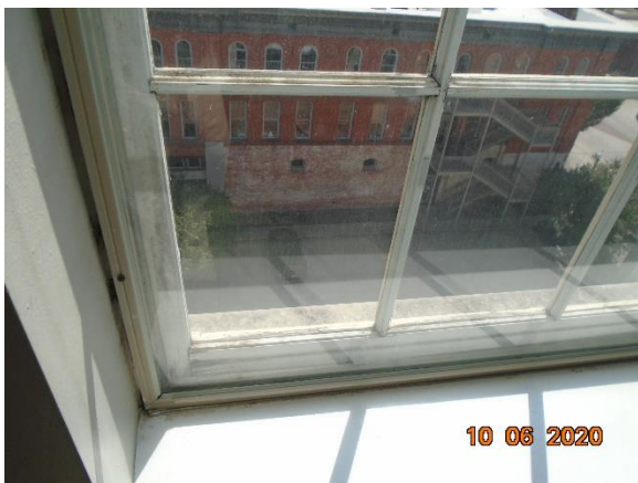
Interior view of interior storm window system and Wood sash with moisture damage
