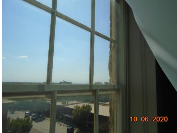
Window mullions loose
