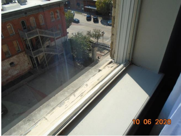
Exterior wood sill water damage/deterioration
