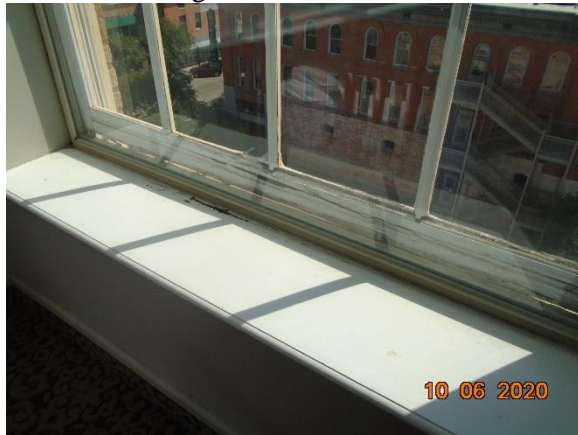
Interior guest room window with damage
