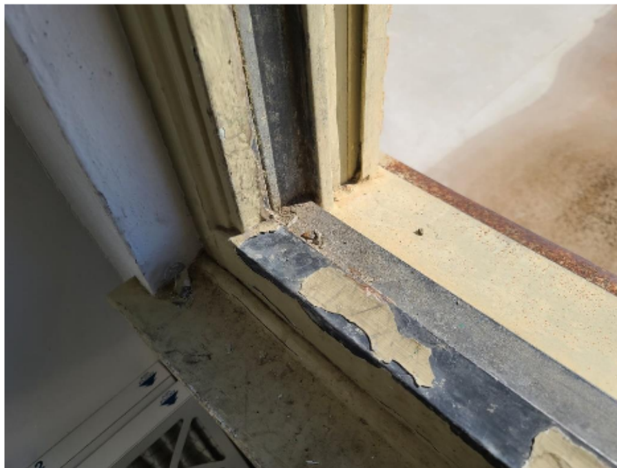
Note the similar “almost flat” sill, and how it is extended over the cast stone sill. The “almost flat” cast stone sill and steel frame does not deteriorate due to water accumulation; whereas a wood framed window sill would be subject to rot)
