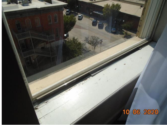
Interior wood window sill water damage
