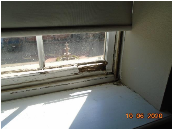
Interior – rotten window sash
