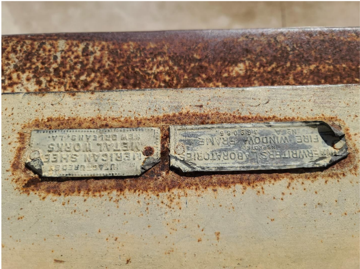
Manufacturer's metal labels on the steel framed window sill in the Varisco Building.
