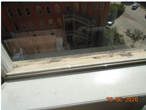
Another view of exterior window sill rot
