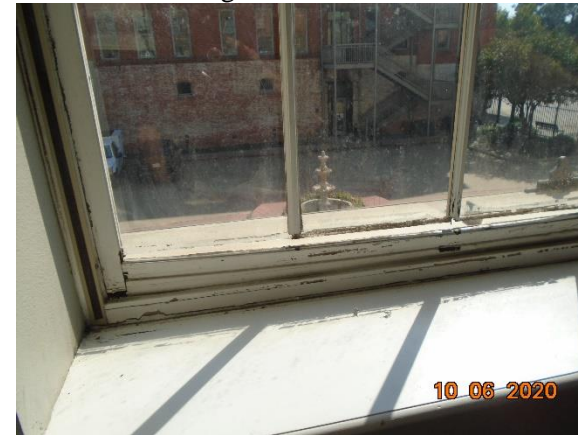
Interior – sash and sill damage
