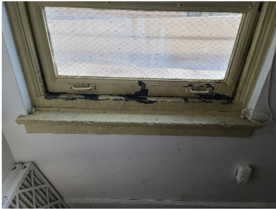
One of the windows on the south side of the Varisco Building. This window is still operational. (Note the similar appearance and condition of the La Salle Hotel steel framed windows.)
