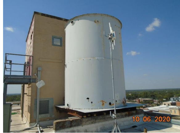
Roof mounted water tank, not in use, has rust.
