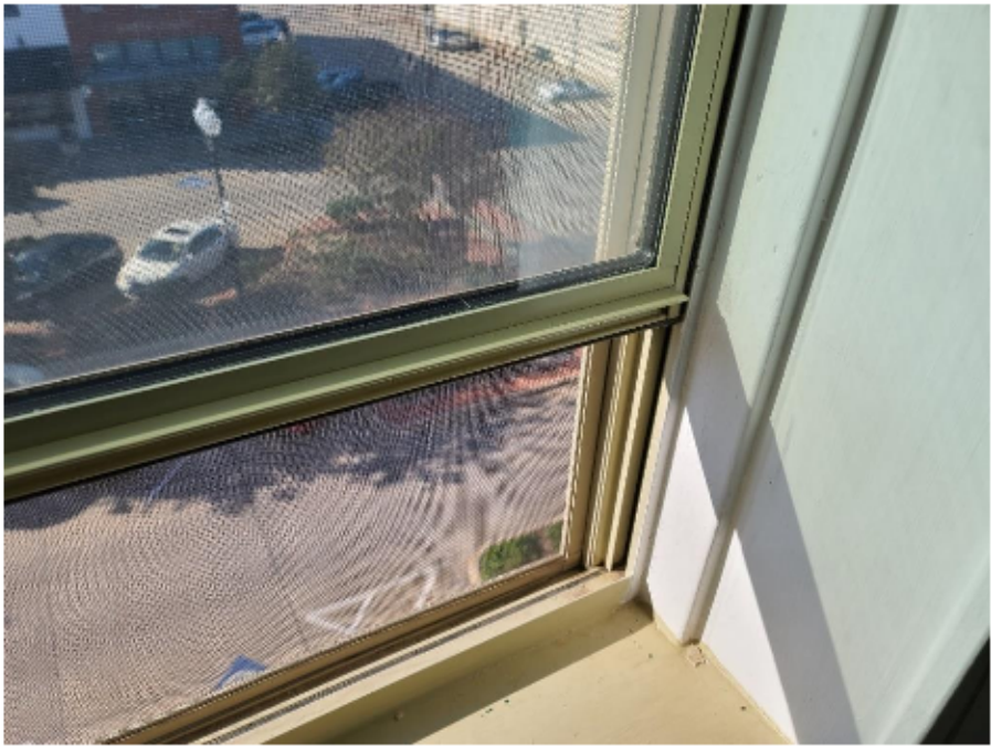
Sill/frame conditions of a typical paintable composite framed window in the Varisco Building (these replaced the steel framed windows in the late 90's.)
