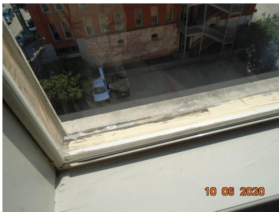
Window opening missing wood sashes and with only interior storm window
