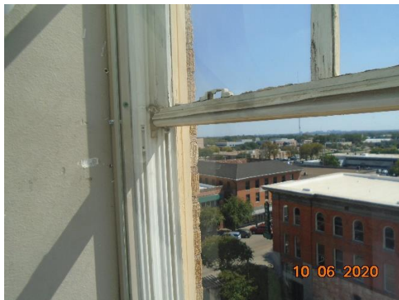
Window missing lower wood sash
