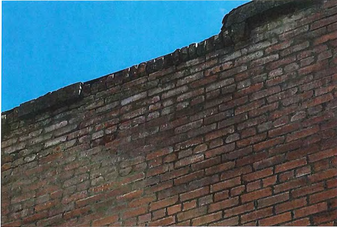
Detail – north wall parapet coping failure, view facing south
