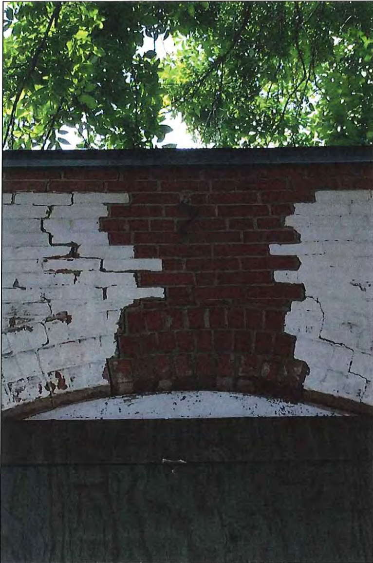
Detail – east wall, previous repair attempt
