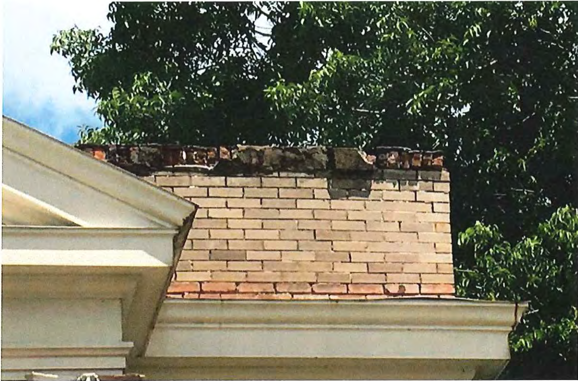
Detail - west wall parapet coping failure
