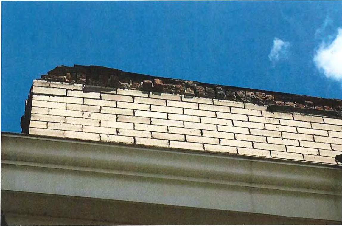
Detail - west wall parapet coping failure
