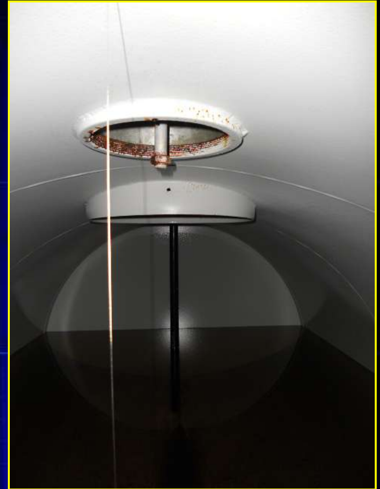
Jet A Tank 2
